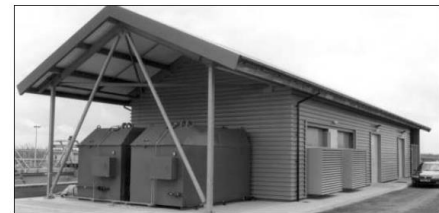
Good example of purpose made building to house two 1000 kVA generators with sound attenuators extending to the outside.
